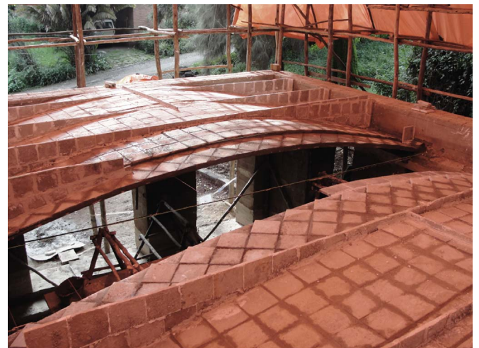
Fig. 6. Thin-tile floor with spandrel walls of the SUDU project in Addis Ababa, Ethiopia, 2010 [13].
